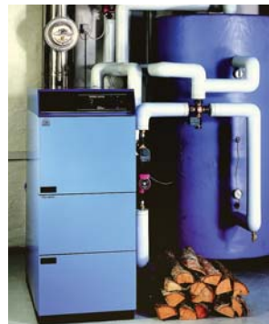
A heat storage system will produce and store hot water throughout the year.
