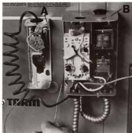
Connecting overheating control (A) and master hot-water control (B) normally requires skill of a professional.
