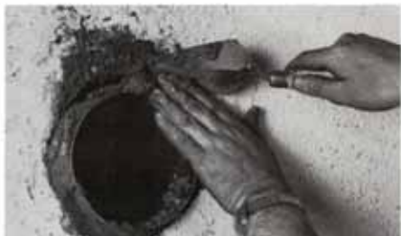
Before flue pipe was passed through wall, thimble was mortared in place. Then flue pipe was inserted and the joint sealed.
