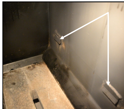
Fig. 4.11 Primary Air Ventilation Holes
